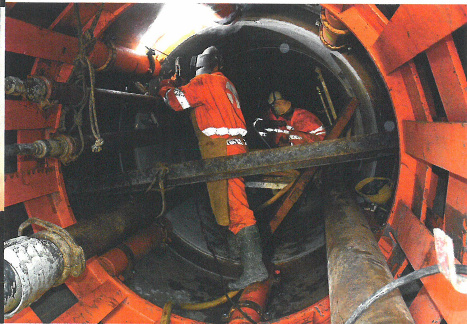
Construction of the Tamazunchale project, some 150 miles northeast of Mexico City, required boring a tunnel through a mountain to lay the 30- and 36-inch pipeline.
